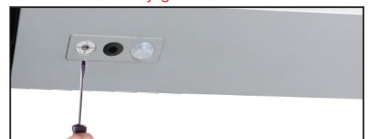
Motion Sensor & Daylight Sensor
